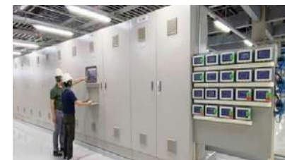
Energy-saving system for the chilled water system
