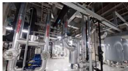
The hot water system was switched from an electric boiler to a gas boiler to reduce carbon emissions
